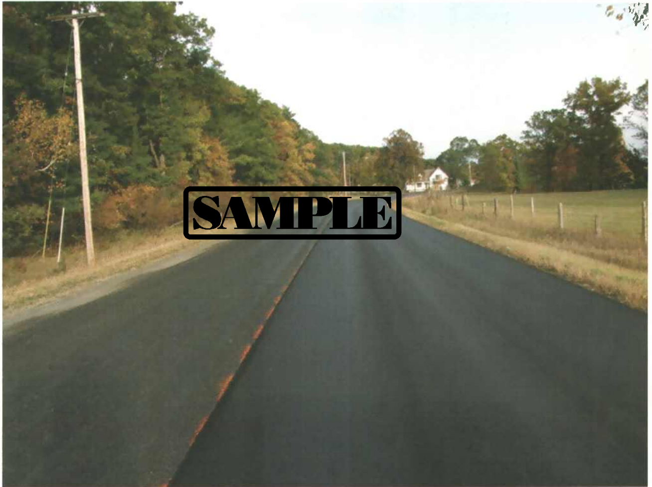
The ultra thin mix specified (right lane) for the project is a commercial ADT (average daily traffic) design requiring a PG 64-28 polymer modified binder. The left lane illustrates how the Hot In-Place process rejuvenates an aged pavement.
